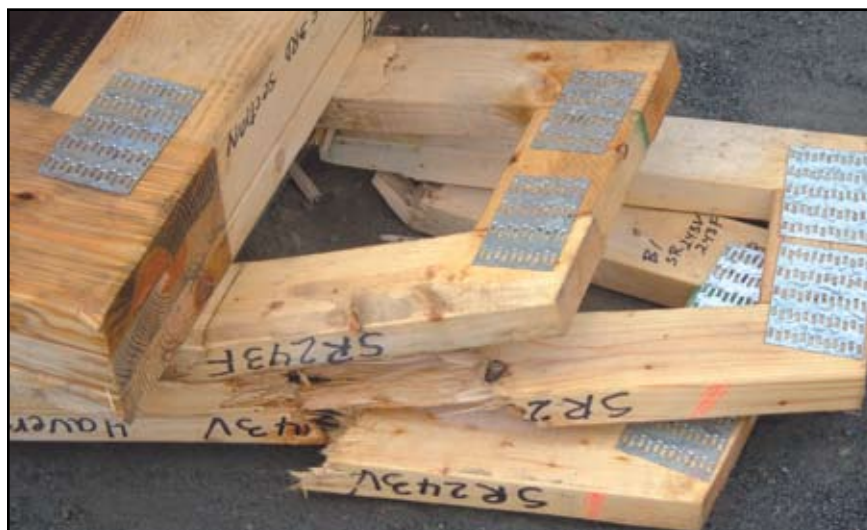
Figure 2: Damage to the ends of three trusses resulting when additional trusses were dropped on top of them during delivery.
